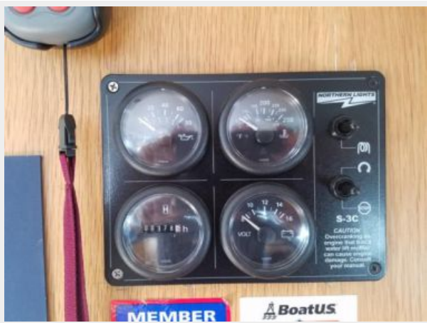
Broadblue 435ST generator instruments
