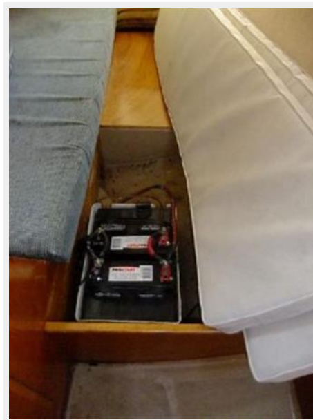
Beneteau 285 - Aft Berth Under Storage - House & Starter Batteries
