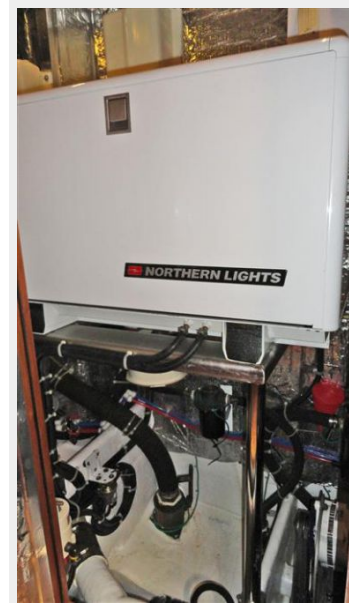
Engine Room, Aft
