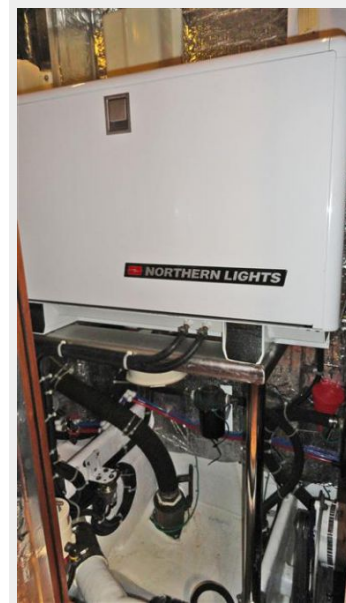
Engine Room, Aft
