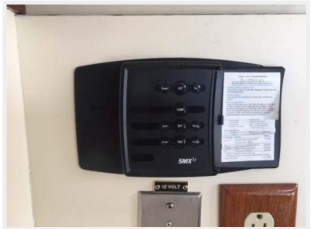
Heat/Air Control Panel
