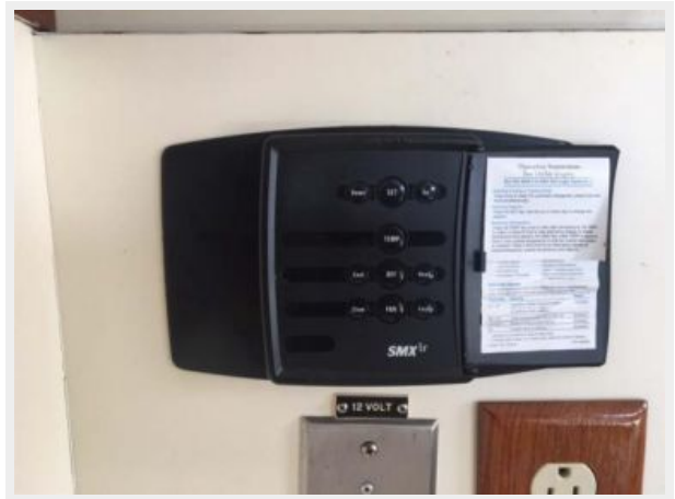
Heat/Air Control Panel
