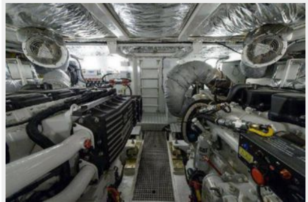
60 Princess Engine Room
