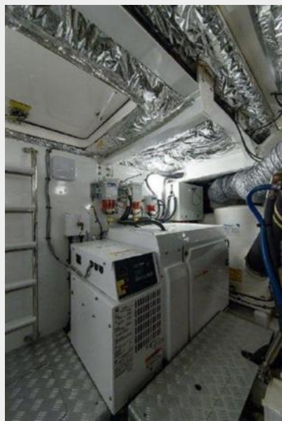
60 Princess Engine Room
