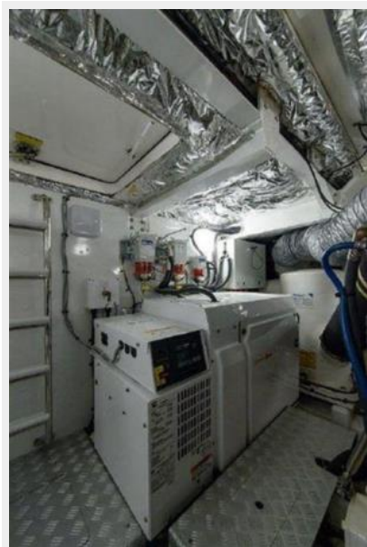
60 Princess Engine Room
