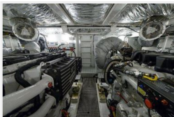
60 Princess Engine Room
