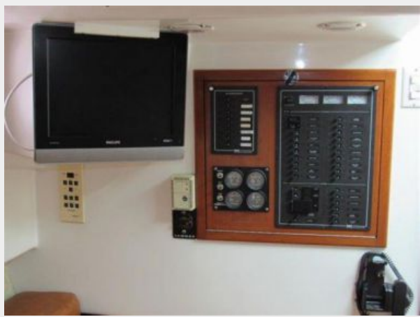
Main Cabin 6 - TV & Electrical Panel
