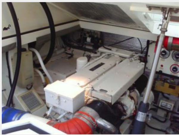
Engine & Mechanical Equipment 4 - Port Engine
