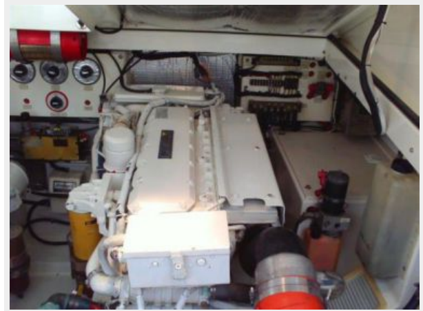
Engine & Mechanical Equipment 5 - Starboard Engine
