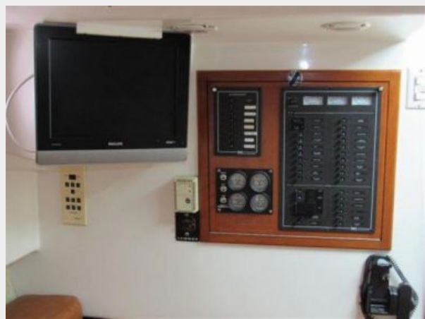
Main Cabin 6 - TV & Electrical Panel
