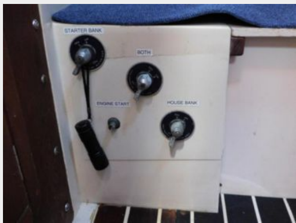
71 42&apos Catalina battery switches
