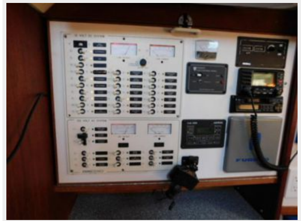
52 42' Catalina electrical panel a.
