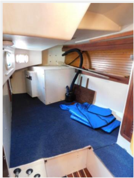
42 42&apos Catalina cabin 3 storage generator
