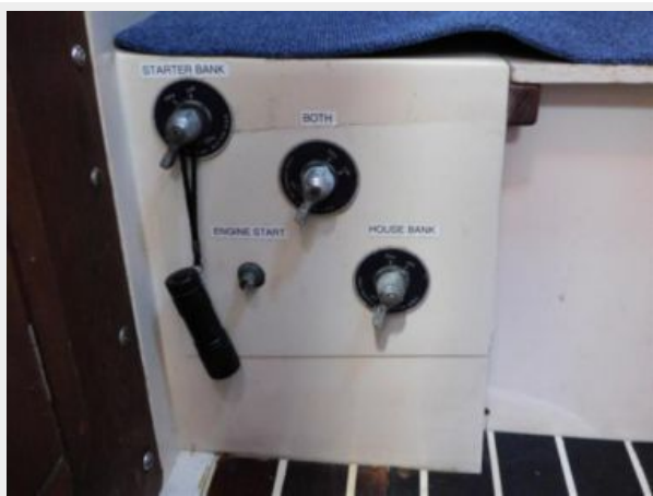
71 42&apos Catalina battery switches
