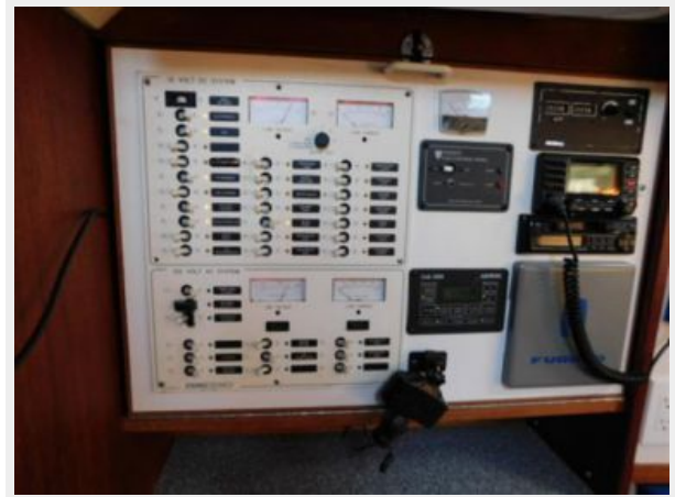
52 42' Catalina electrical panel a.
