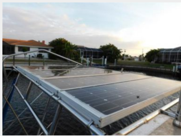
18 42' Catalina solar panels
