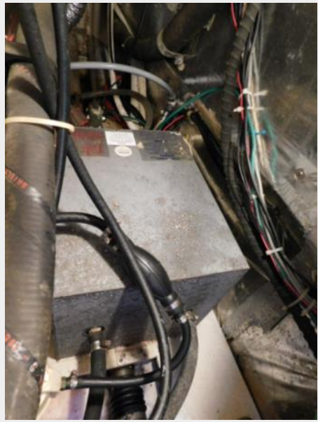
54 42' Catalina water heater
