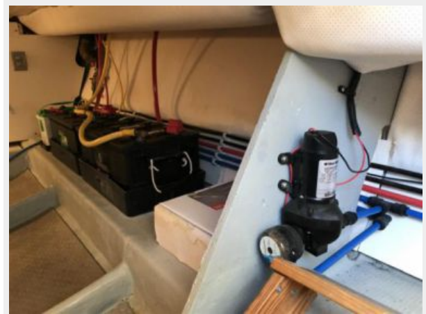
311 Battery and Water Pump
