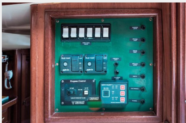
2nd Sub panel at Entry, lights & Bilge
