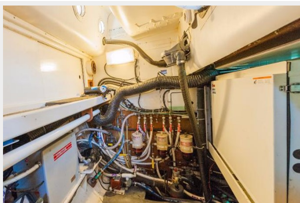
Standup Engine room - well planned
