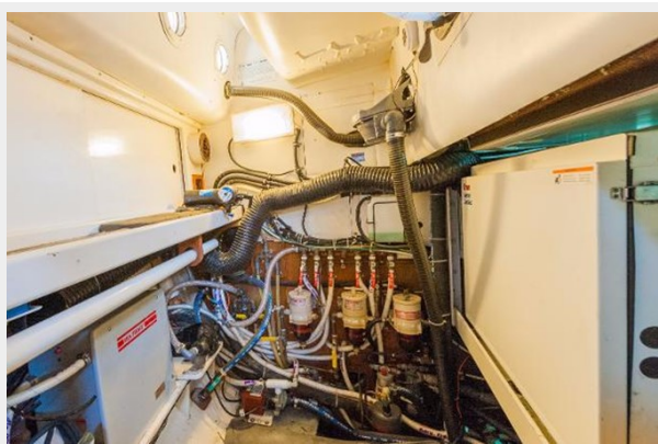
Standup Engine room - well planned
