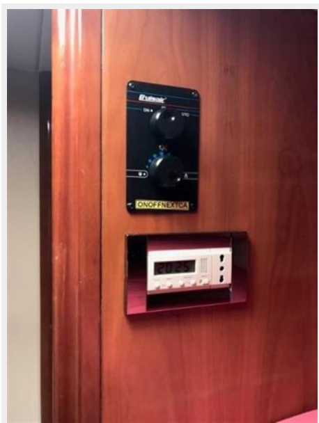
Stateroom Airconditioning Controls
