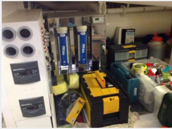
Engine Room Detail
