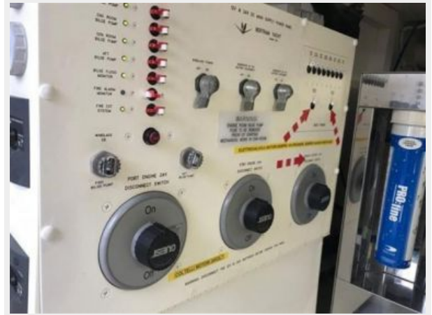
Engine Room Battery Switch Panel
