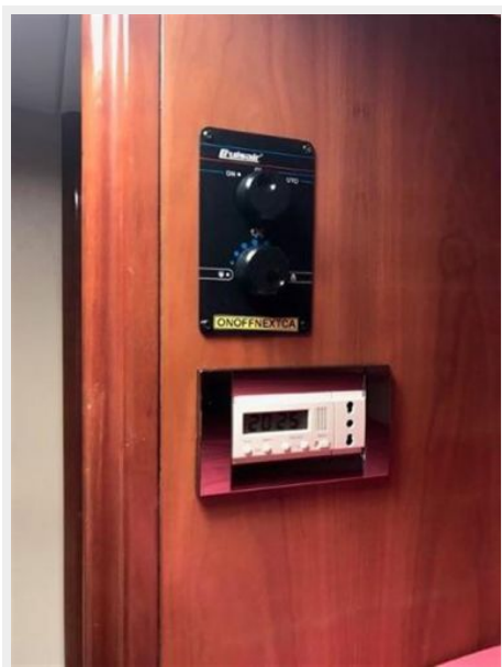
Stateroom Airconditioning Controls
