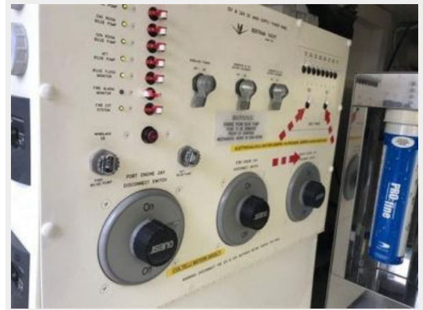
Engine Room Battery Switch Panel
