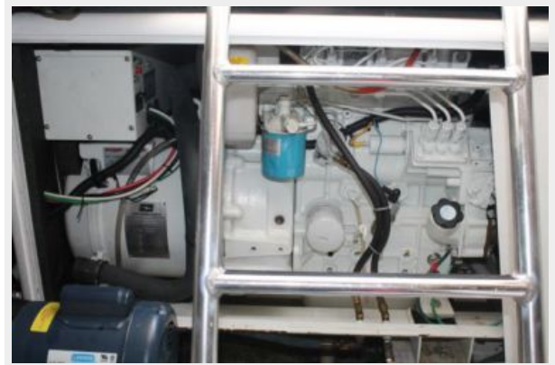
Northern Lights Generator
