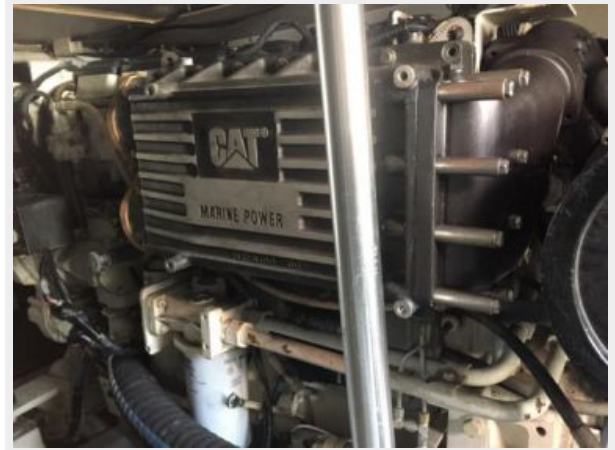
New After Coolers 4.10.18
