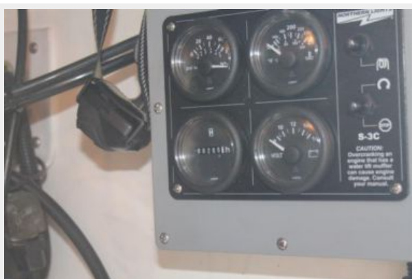
Northern Lights Generator
