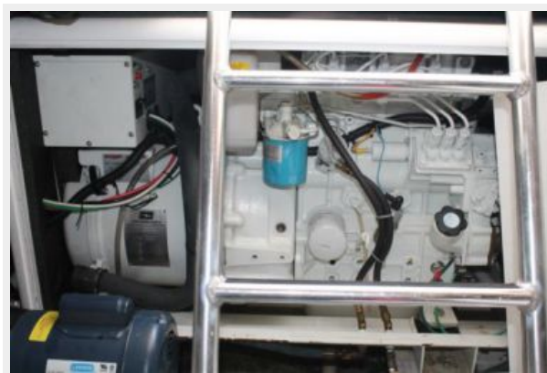
Northern Lights Generator
