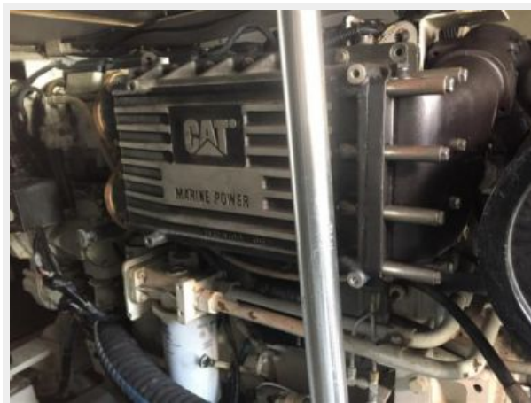
New After Coolers 4.10.18
