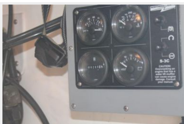
Northern Lights Generator
