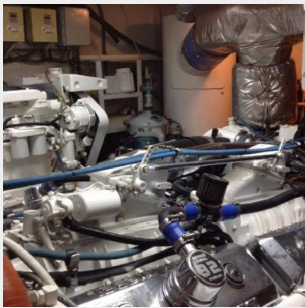
ENGINE ROOM - Looking to Sbd Side & U/W Exhaust
