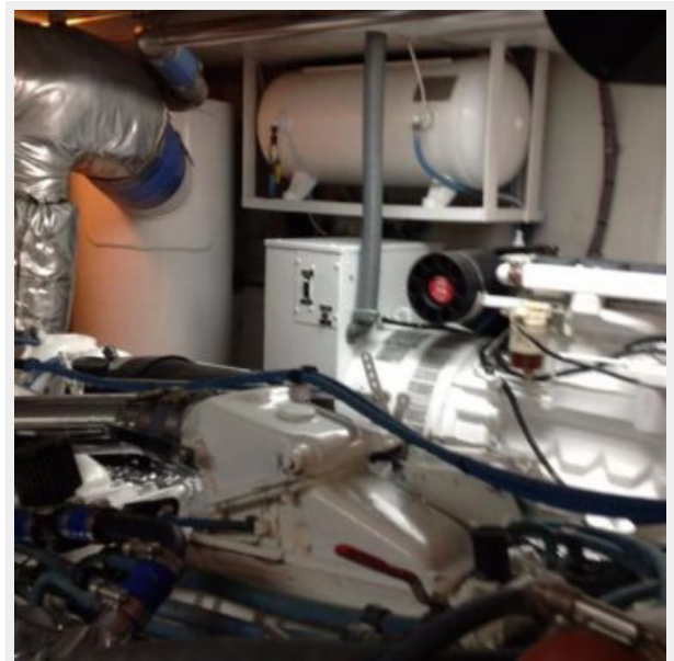
ENGINE ROOM - Looking at Port Side
