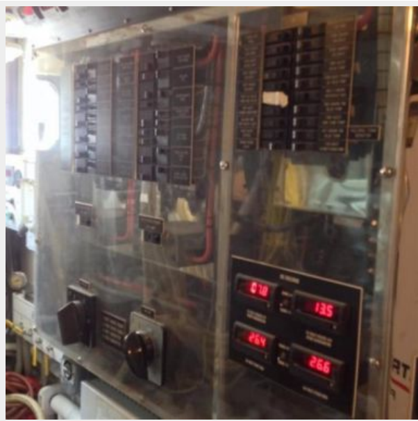
ENGINE ROOM - Main Electrical Panel
