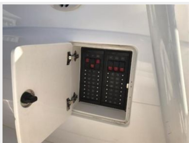
327 Intrepid | Battery switches panel
