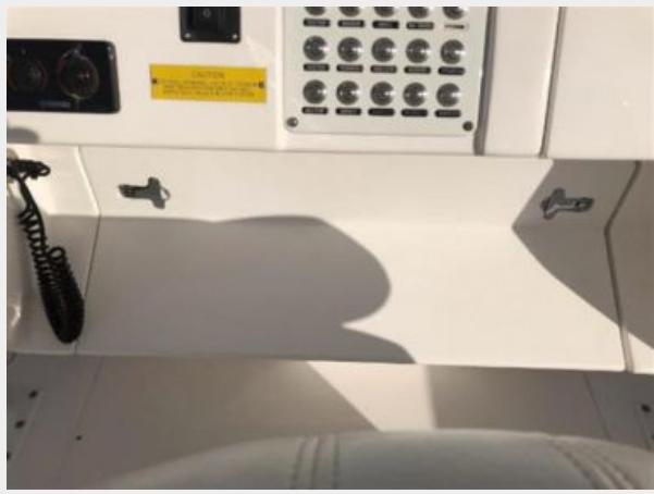
327 Intrepid | Battery and breaker location
