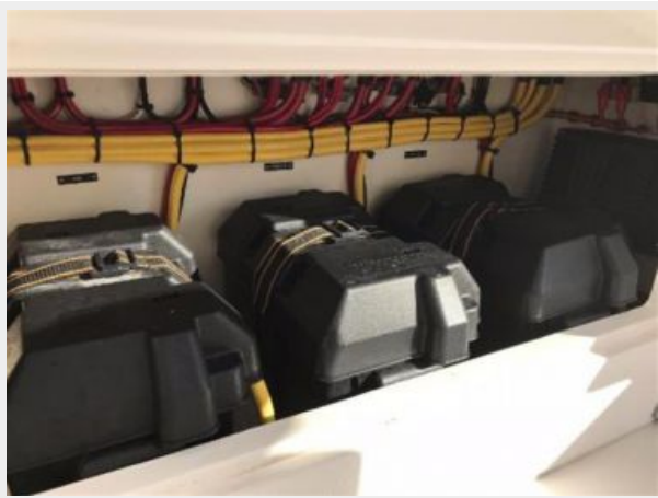
327 Intrepid | Battery boxes
