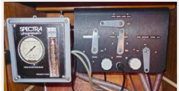
Water Maker Controls
