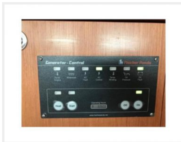
Generator panel with 692 hours
