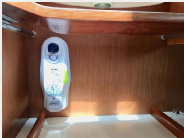
EPIRB mounted under the companion way entrance
