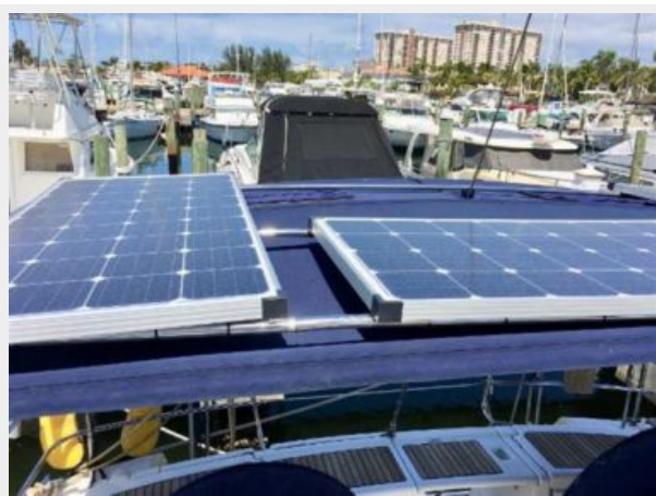
Solar panels on a rack over the Bimini frame 480 Watts new in 2018
