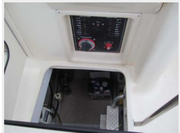
Engine Room Access
