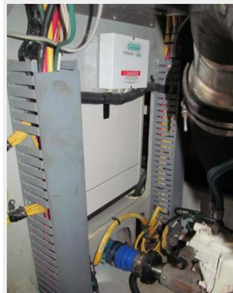
Engine Room Wiring Protection
