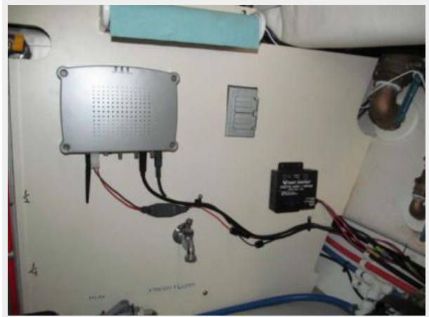
Engine Room Starboard Aft
