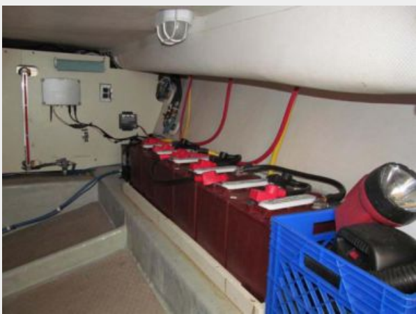
Engine Room Starboard Side
