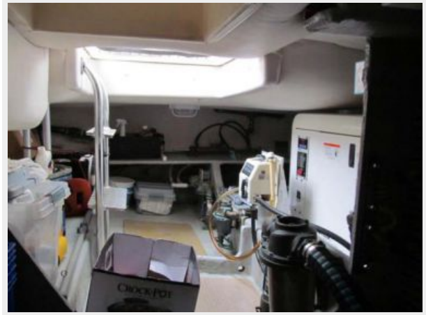
Engine Room Aft
