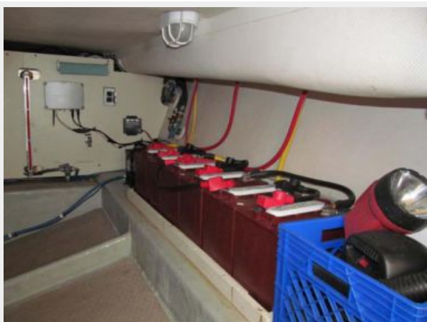
Engine Room Starboard Side
