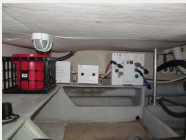
Engine Room Port Aft
