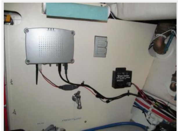
Engine Room Starboard Aft
