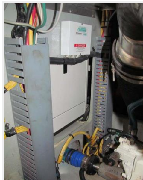
Engine Room Wiring Protection
