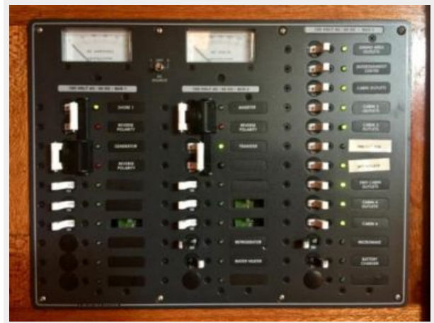
AC/DC Breaker Panel
