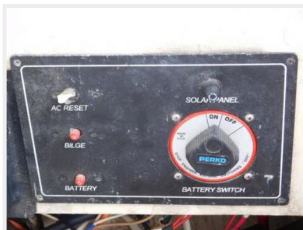
Solar Panel Power Switch
