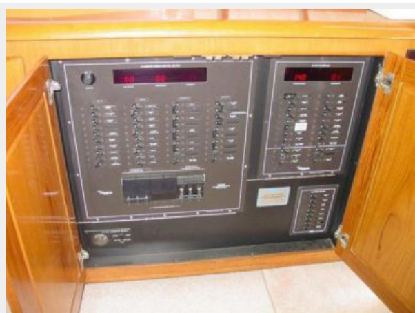
Salon 4 - Electrical Panel
