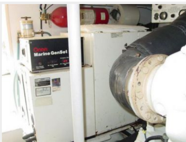
Electrical System / Equipment - GenSet
