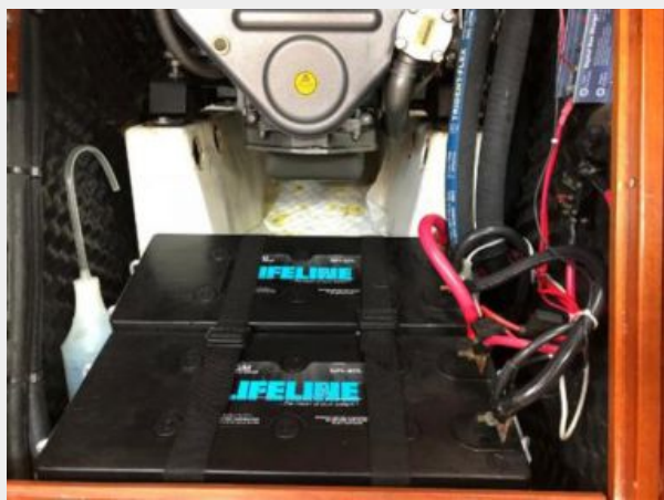
Two 4D AGM batteries
