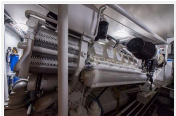
Engine & Mechanical Equipment 2
