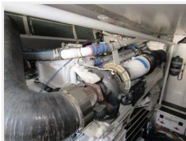
Engine & Mechanical Equipment 4
