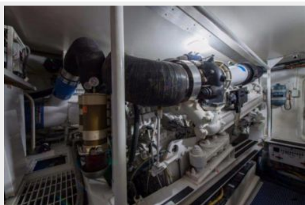
Engine & Mechanical Equipment 3
