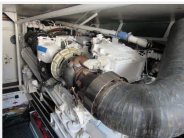
Engine & Mechanical Equipment 7
