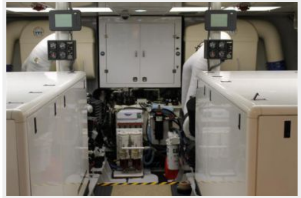
Engine Room Looking Aft
