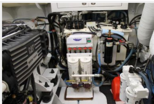
Engine Room Looking Aft
