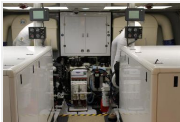
Engine Room Looking Aft
