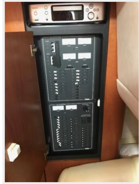
Main Distribution Panel
