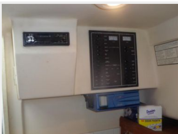
Electrical System / Equipment 1
