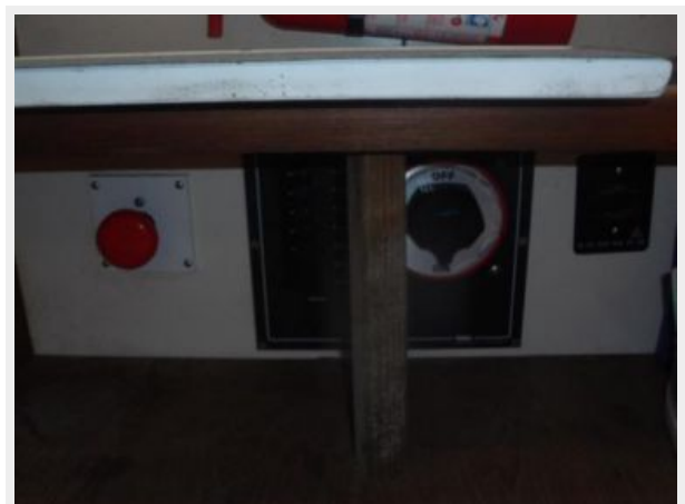
Electrical System / Equipment 2
