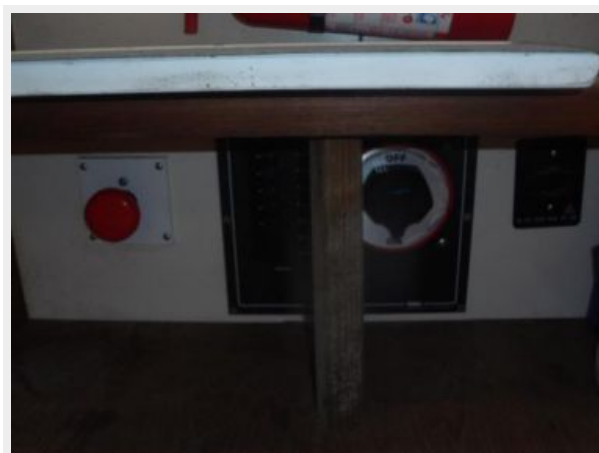
Electrical System / Equipment 2
