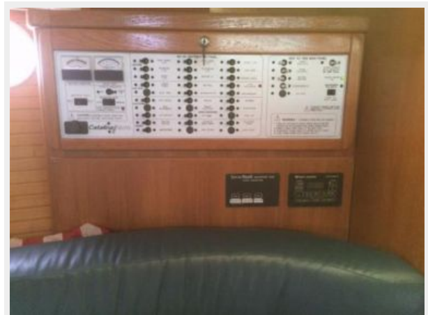
AC / DC Panel, Inverter
