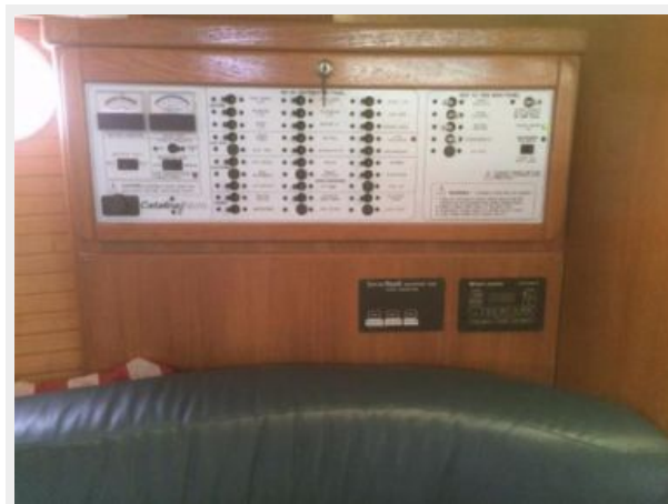
AC / DC Panel, Inverter
