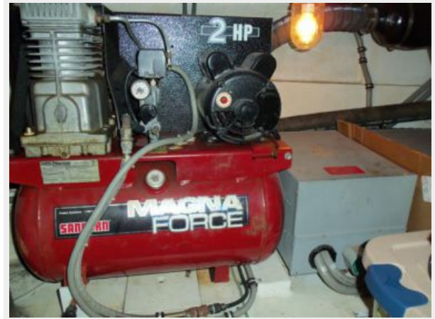
Starboard Side Gen Room
