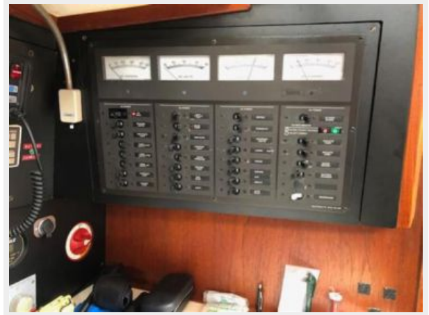
Breaker panel for DC/AC voltage
