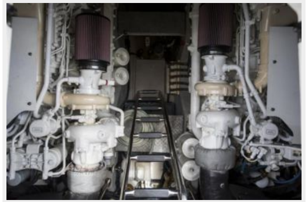
Engine room view 1
