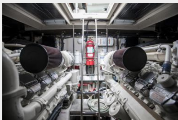
Engine room view 2
