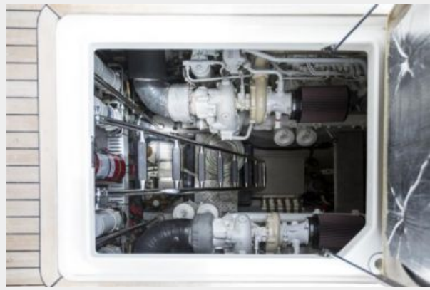
Access to the engine room
