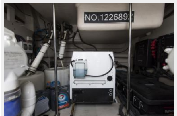
Engine room view 3
