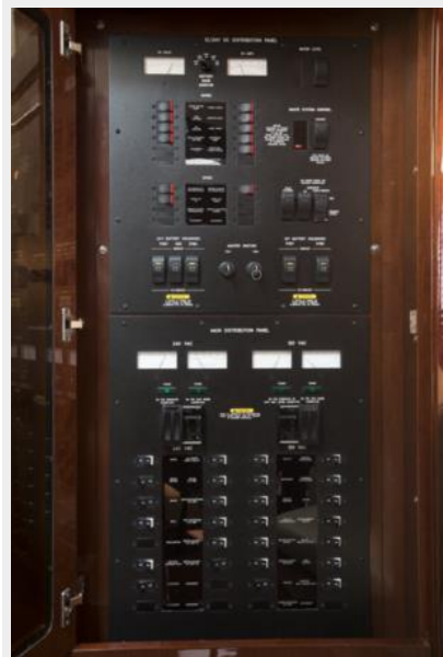
Main distribution panel
