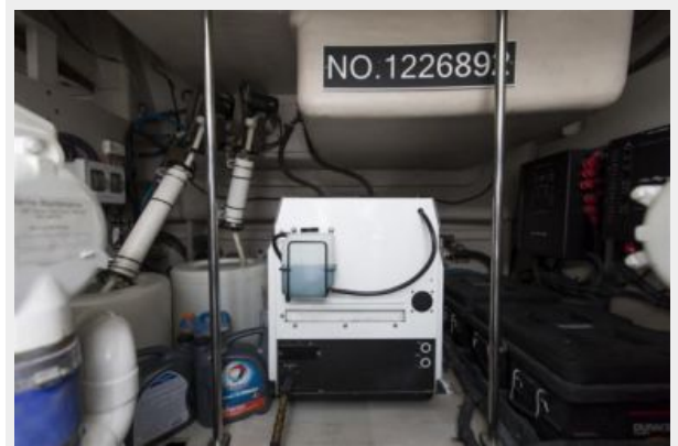
Engine room view 3
