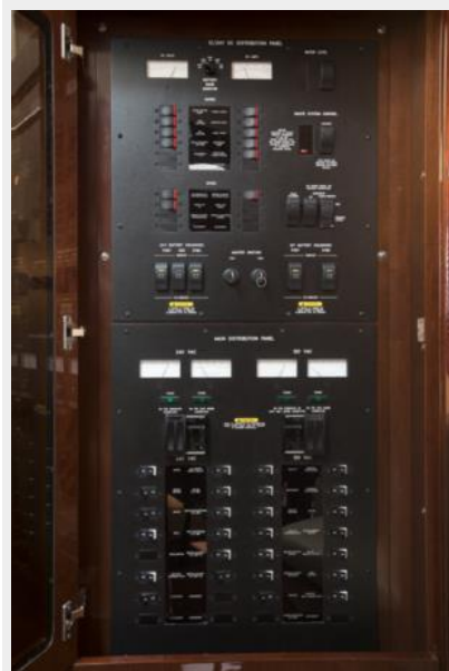
Main distribution panel
