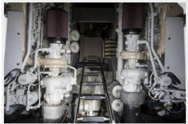
Engine room view 1
