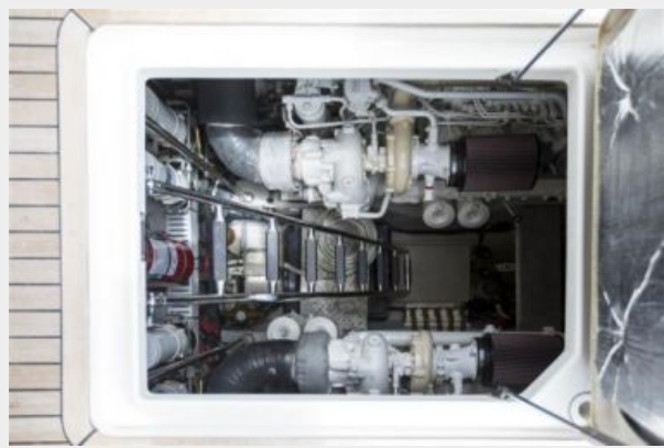
Access to the engine room
