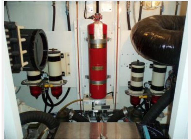
Engine Room Center
