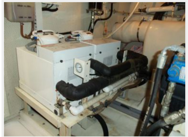
Chilled Water AC
