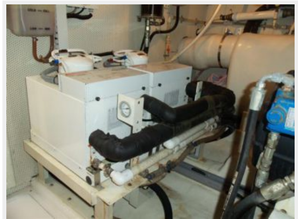
Chilled Water AC
