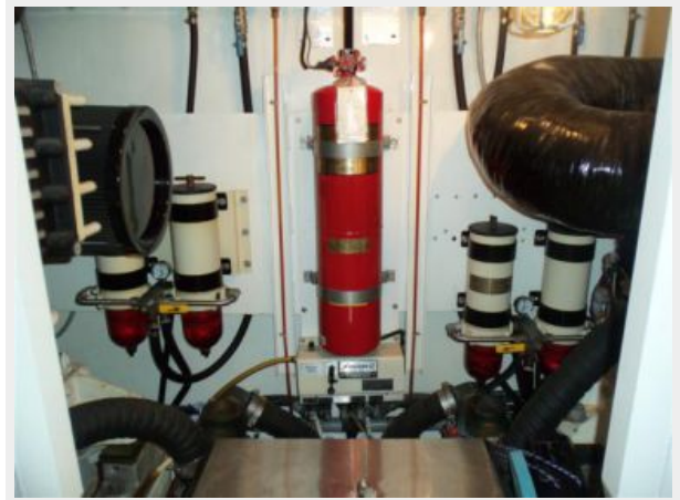
Engine Room Center
