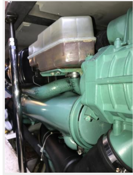
360 Carver SS - Engine Room
