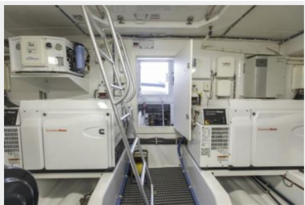
Engine room view 2
