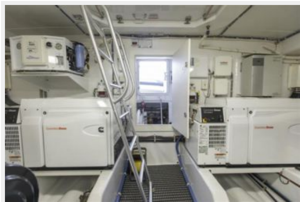
Engine room view 2
