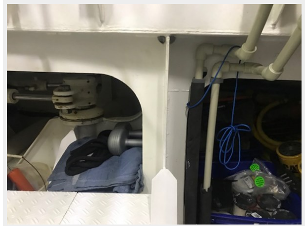
Lazarette bildge under floor plates 3
