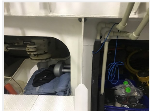
Lazarette bildge under floor plates 3
